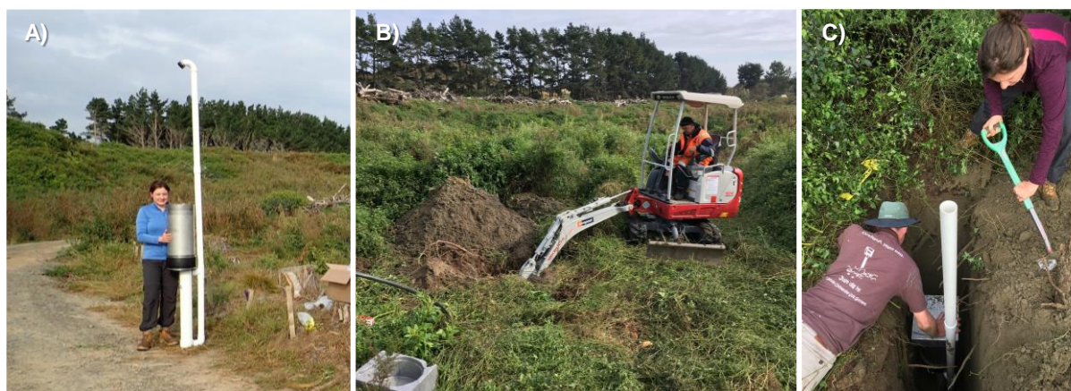
Figure 8 A) Water flux meter (WFM) ready for installation; B) Digging the trench for the installation of the WFM; C) installing the WFM.
